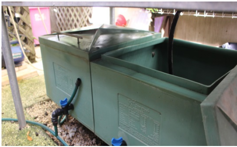
The new 150 L supply tank
