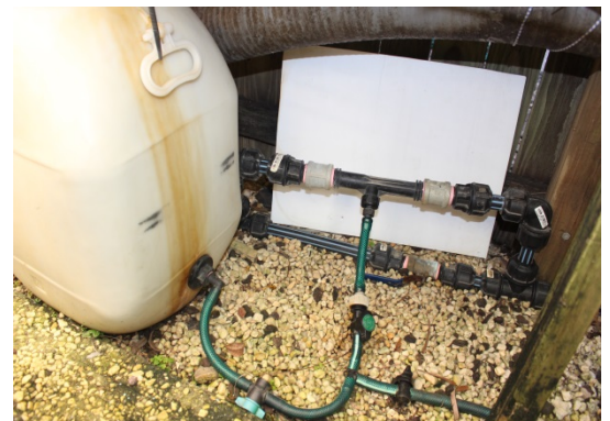
The 20 L supply tank and connections
